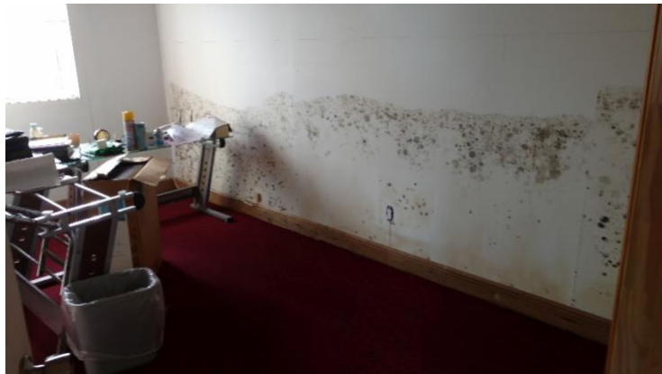
Mold growth shows the 4-ft water line inside Caravel Zion
