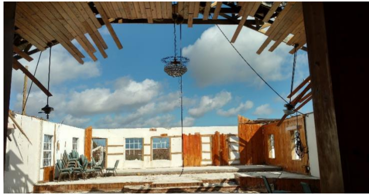
One of the more severely-damaged churches
